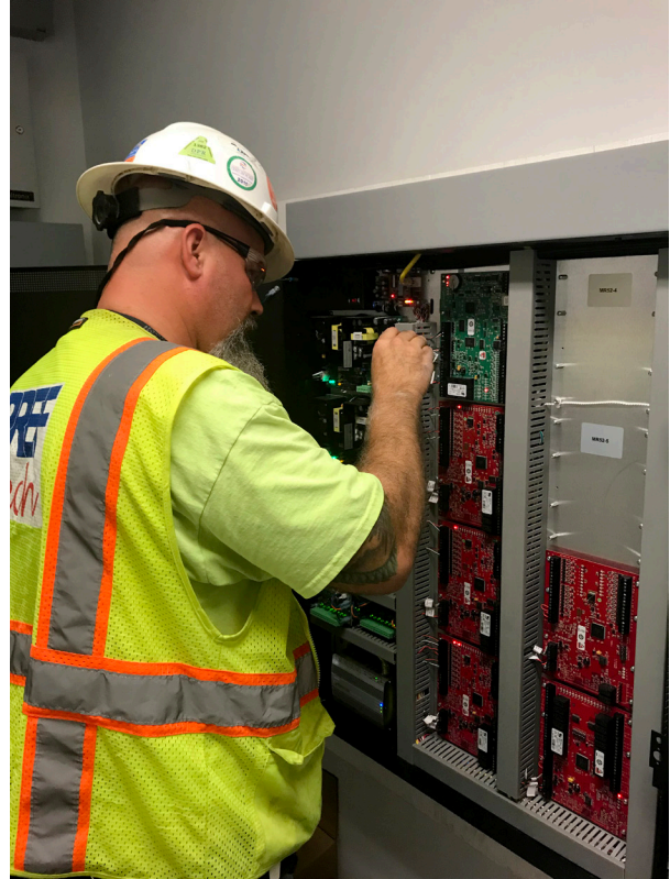
P ref-Tech Lead Technician/Superintendent Ryan Nelson tests the newly installed ProWire solution for Travis County.
